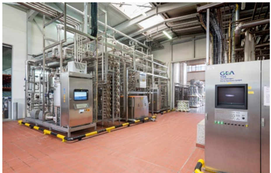
The new GEA infusion plant for ESL milk production was connected to the automation system Tetra Pak PlantMaster (photo: Hohenloher Molkerei)
