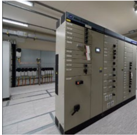
Arranged in 42 cabinet columns, the MCC installation is 50 m in length (photo: Rockwell Automation)
