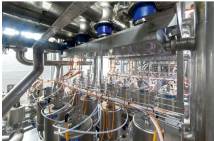
The new valve knots in the milk intake and/or for the milk storage facility make production even more flexible (photos: Hohenloher Molkerei)
