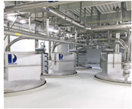
A total of 13 powder silos was installed at MILEI (photo: Derichs)
