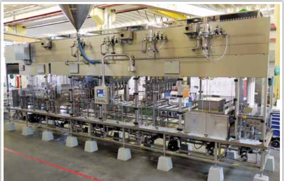
This Waldner filling line using pulsed light cup sterilization is operating at Weissenhorner Milchmanufaktur in Germany (photo: Claranor)
